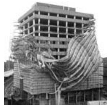
Sheeted scaffolds incur higher wind loading
